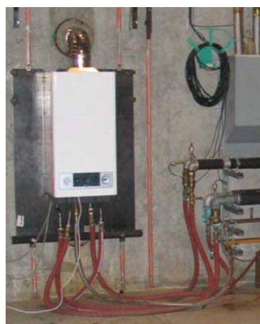
Boiler under test.
